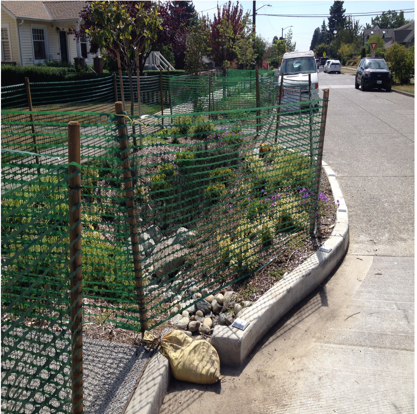
Sand bags prevent silt-laden flow from entering the bioretention BMP. Green construction fencing prevents compaction due to foot traffic.
