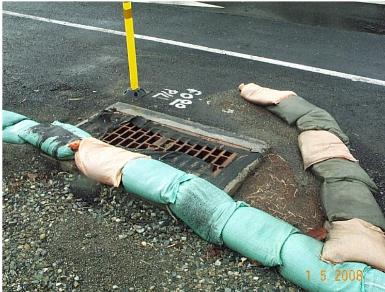
Temporary sand bags divert construction site stormwater runoff to inlet protected with a catch basin filter sock.
