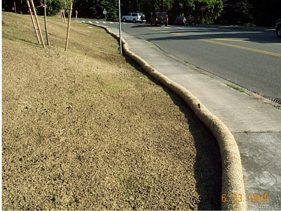
Example of shallow gradient slope with berm installed at downgradient edge to minimize silt-laden runoff onto the sidewalk.
